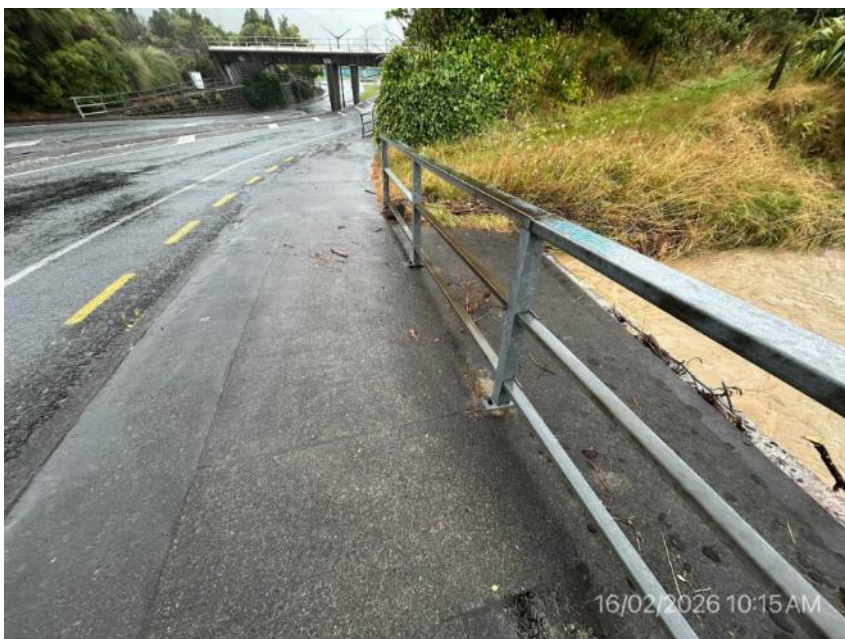
Figure 22 The Field Street road culvert reached full capacity
