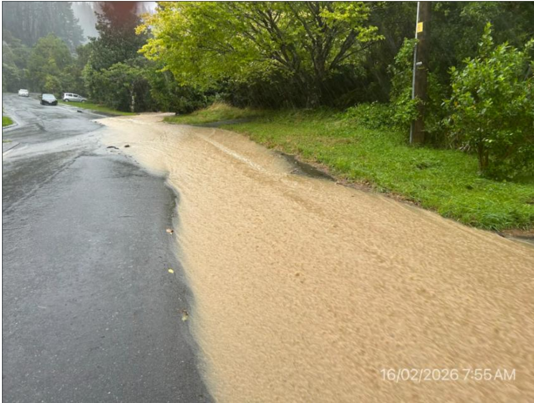
Looking south up to 122 Pinehaven Road where water overtops the driveway culvert
