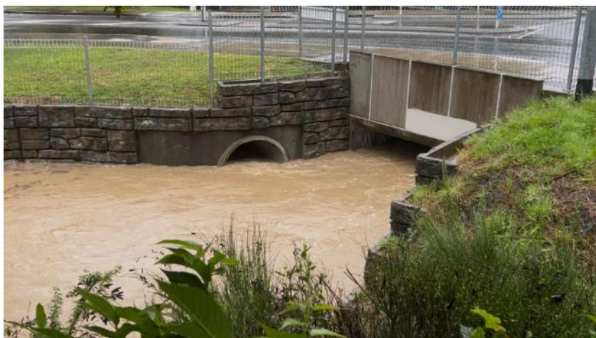
Pinehaven Road culvert: View of the Wyndham Road discharge pipe and the new culvert intake
