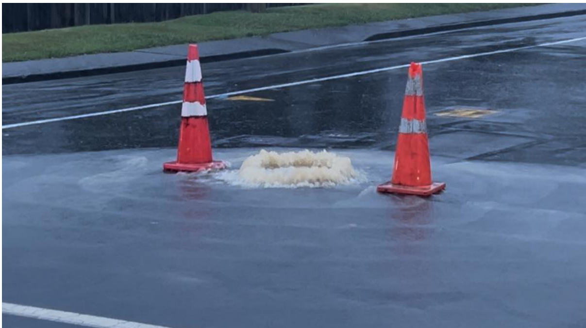
Figure 30 Popped manhole cover at intersection of Pinehaven Rd and Jocelyn Cres (by Library)
