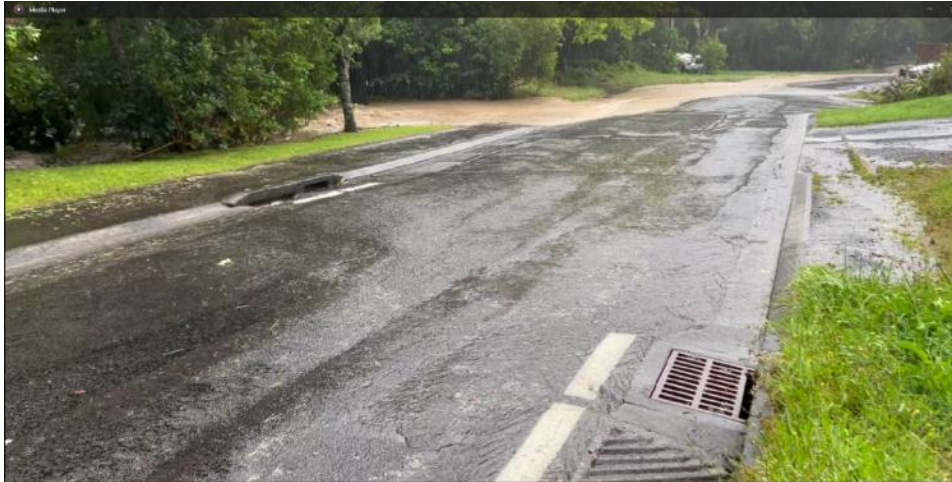
Road sumps contribute to overtopping of culvert at 122 Pinehaven Road
