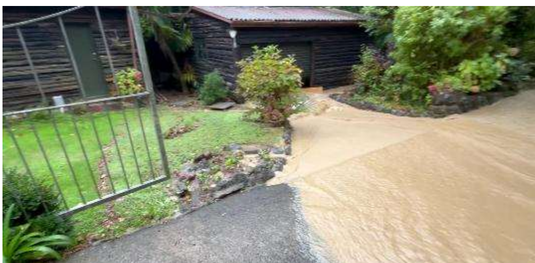
Figure 8 Blocked driveway culvert at 125 Pinehaven Road, 18 April 2026, 10:05am
