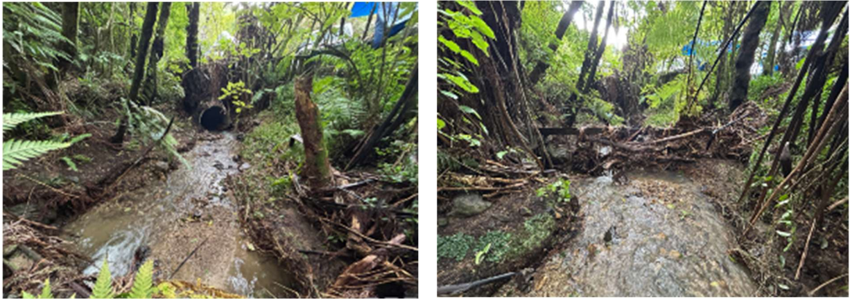
Figure 19 The intake pipe (left, view downstream) and a small debris trap (right, view upstream)
