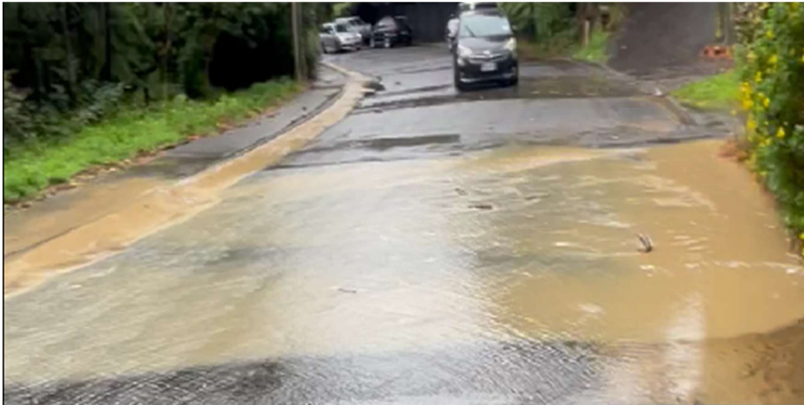
Figure 4 Overtopped culvert near 108A Wyndham Road, 18 April 2026, 9:49am
