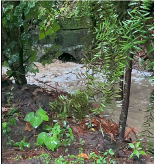
Figure 71 18-4-26 9:55am Public drain discharging into 37 Jocelyn Crescent
