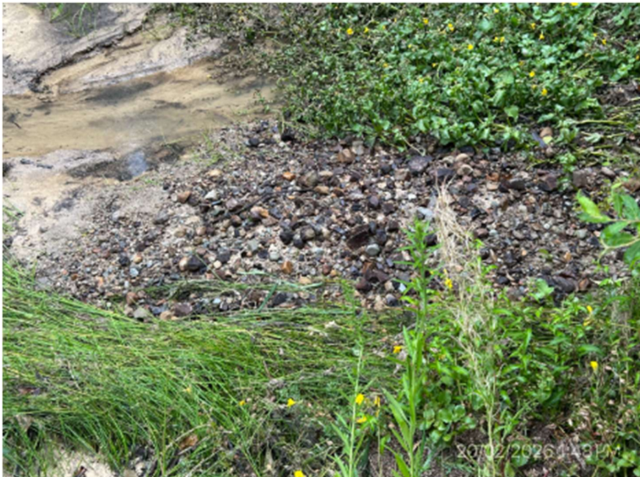
Figure 43 Pioneer Grove culvert, 20 Feb 2026, after storm 16 Feb 2026. Photos: Flooding Us NZ Ltd
