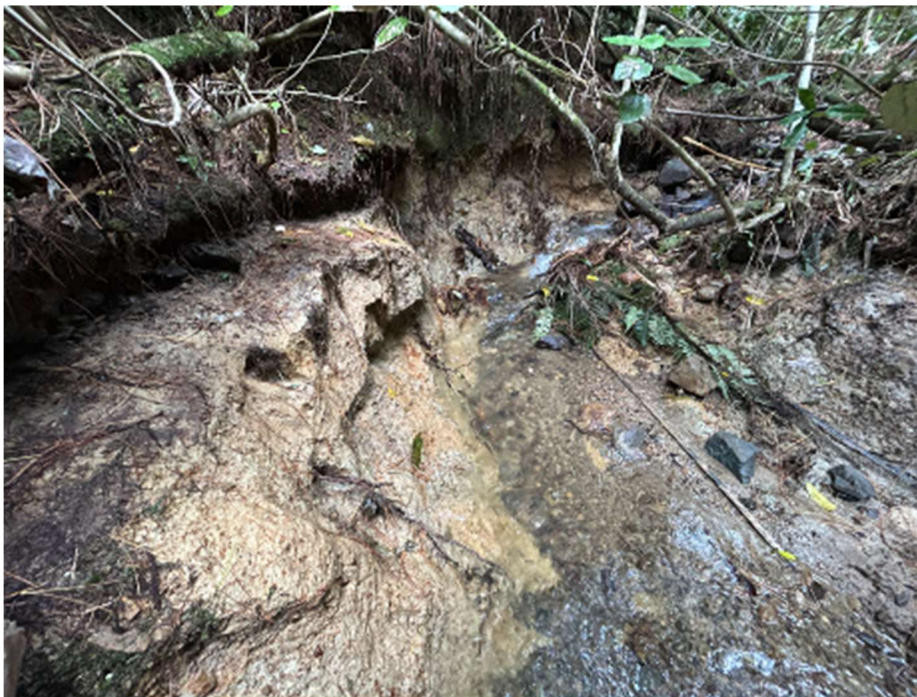
Figure 28 Scouring of the stream banks and bed. Photos: Flooding Us NZ Ltd
