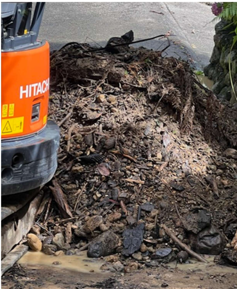
Figure 13 Some of the gravel, rocks and debris removed from the stream channel at 125 Pinehaven Road
