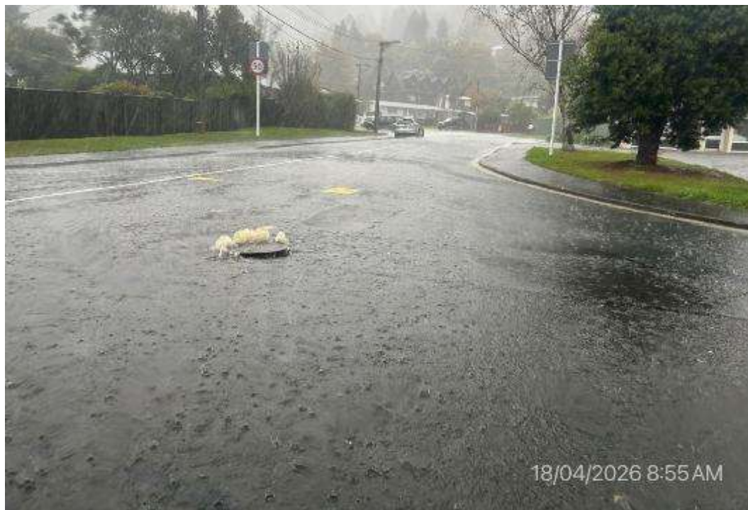
Figure 60 Pinehaven Road and Jocelyn Crescent (north end by Library) wet, but not flooded as shown on GWRC’s 1-in-10-year flood map
