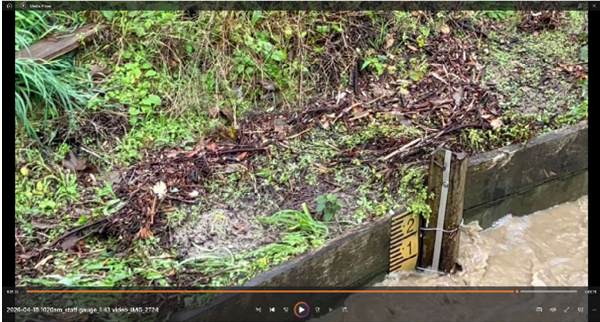
Figure 99 Debris on the bank above the staff gauge on the retaining wall
