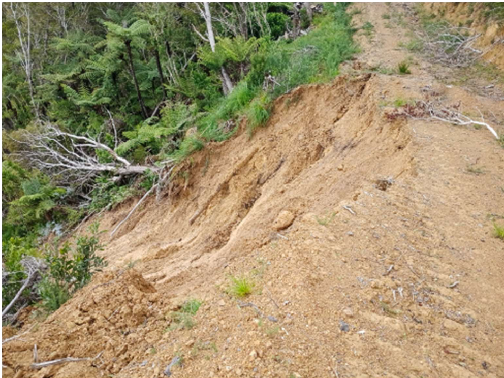
Figure 40 Landslide occurred on edge of GTC logging track (Photo: Dennis Clark)
