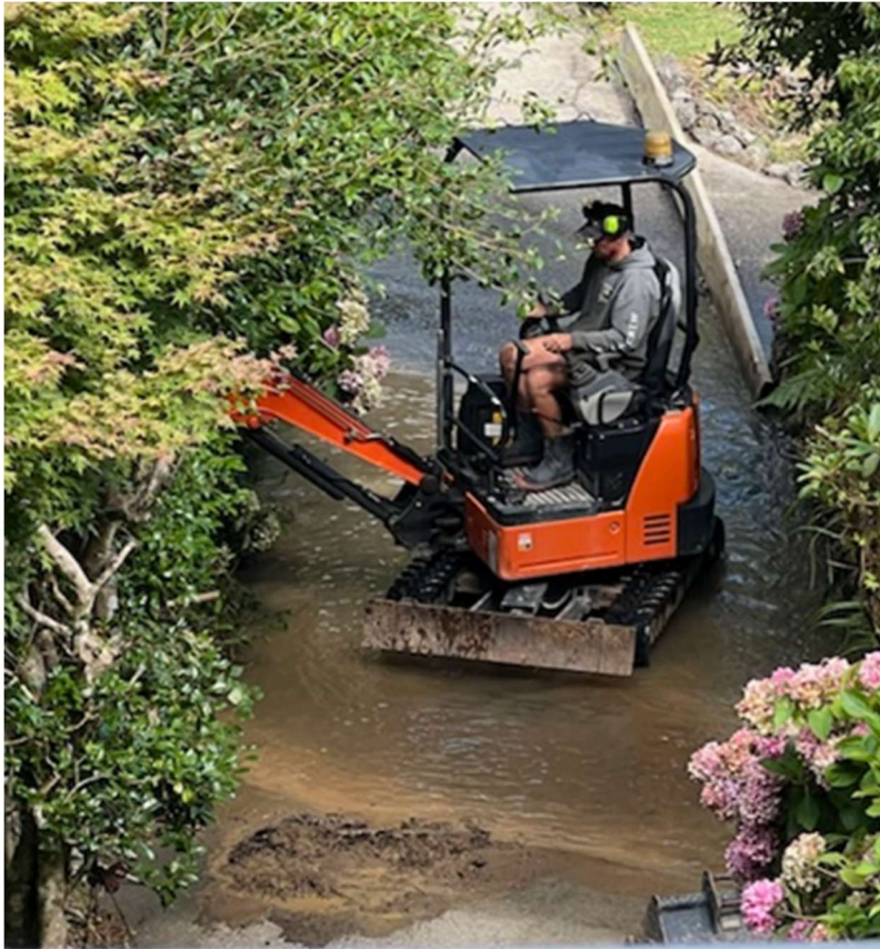
Figure 12 Contractor removed about 30m 3 of gravel and debris from the stream channel at 125 Pinehaven Rd
