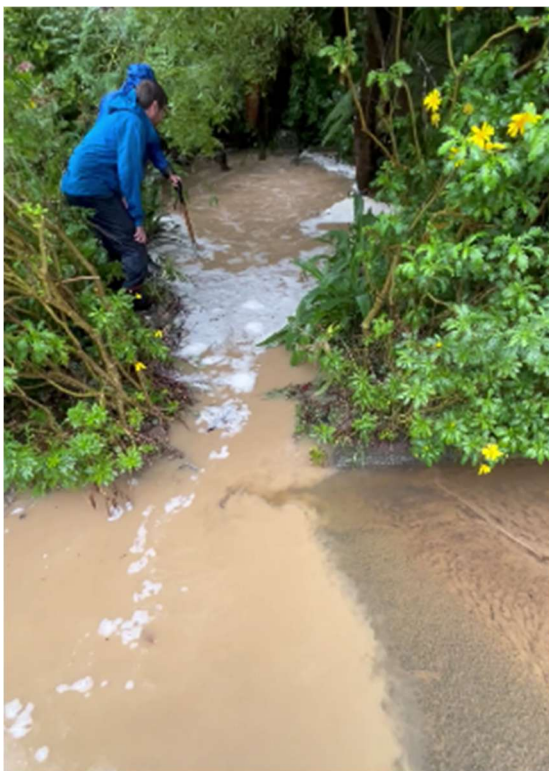
Figure 5 Wyndham Rd culvert blocked, 9:49am
