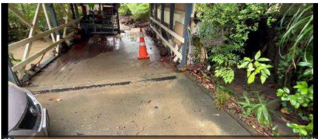
Figure 82 18 April 2026, 10:15am - 30 Blue Mountains Road – water has flooded the bridge
